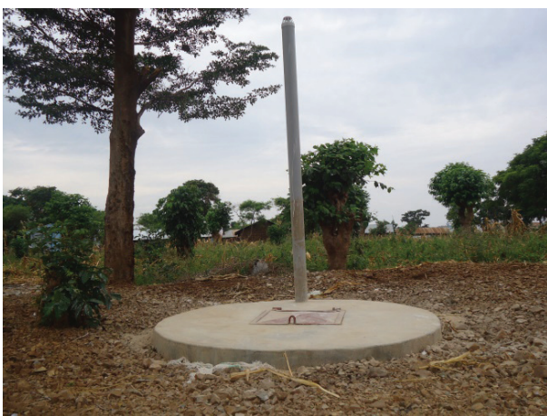
A placenta pit at Hama HC II in Namayingo district-one of the 15 placenta pits constructed at high volume HCs II in the region
